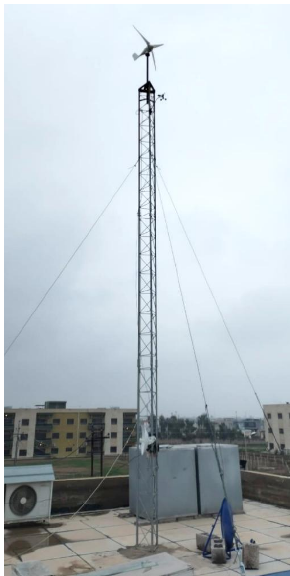
Fig. 7. Vantage Pro2 observed wind turbine setup
